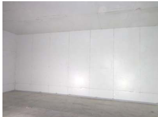
26'1" x 32' x 12' H Drive-In Cooler
